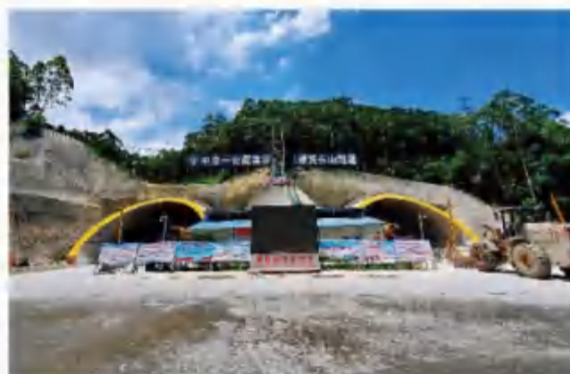
广东省广连高速公路虎头山隧道安全监控 Safety monitoring of Hutoushan tunnel of Guanglian Expressway in Guangdong Province
